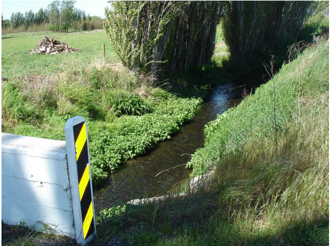
Figure 6: Hanmer Road Drain by Lake Road. This is an example of a well maintained drain that generally has adequate capacity, but where short term flooding occurs following high intensity rainfall. Land in this location was under water for about 12 hours following a storm in 2002.
