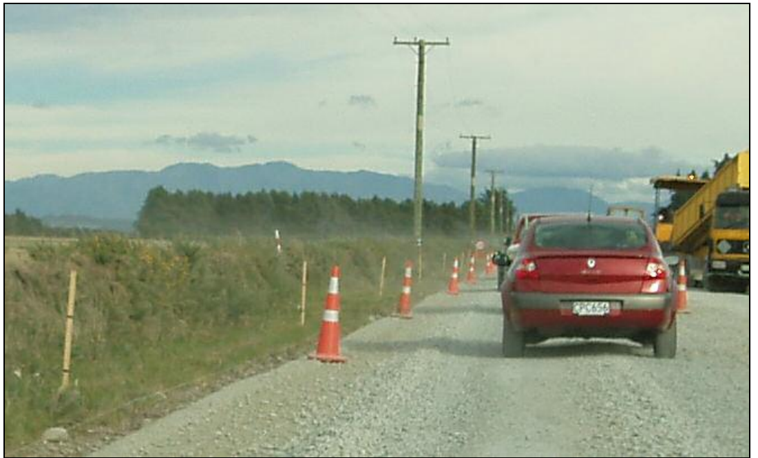
Figure 6 Dust from Roadworks on State Highway 73
