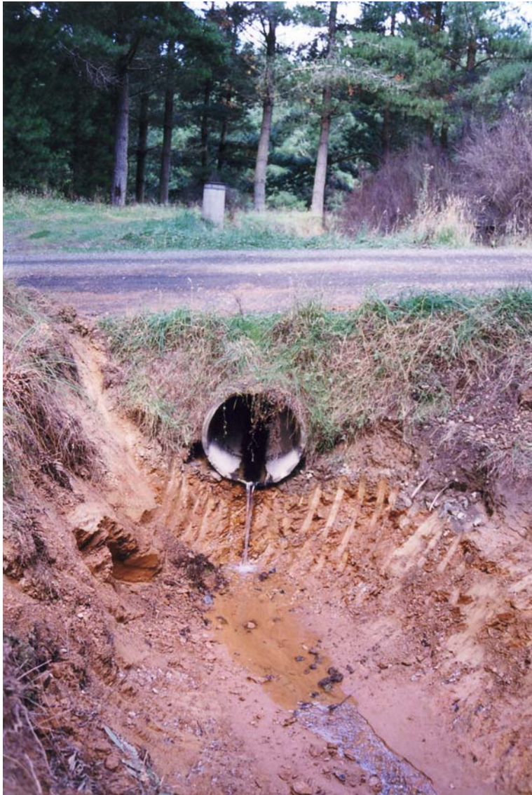
Figure 4. A retro-fitted free fall drop on the Shepherd Stream water race culvert to prevent upstream fish passage.
