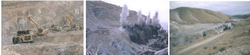
(Fig 7.) Scenes from the construction of the Opuha earth dam, Fairlie. Scenes such as this, blasting, heavy machinery and dust bowls threaten Coalgate.
