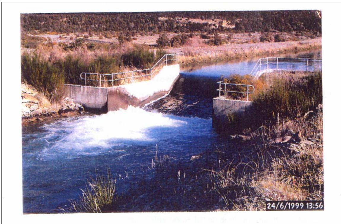
Figure D1: Fish velocity barrier on the Branch River Hydro Scheme's tailrace discharge to the Wairau River
