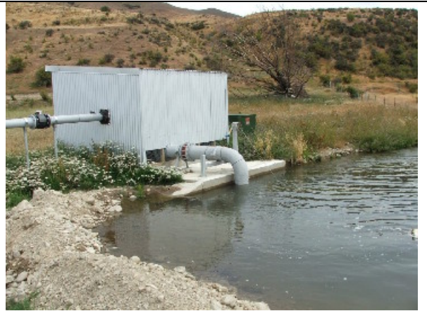
Pump shed from small holding pond at end of race
