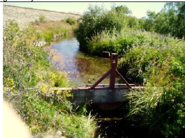
Control gate in diversion channel
