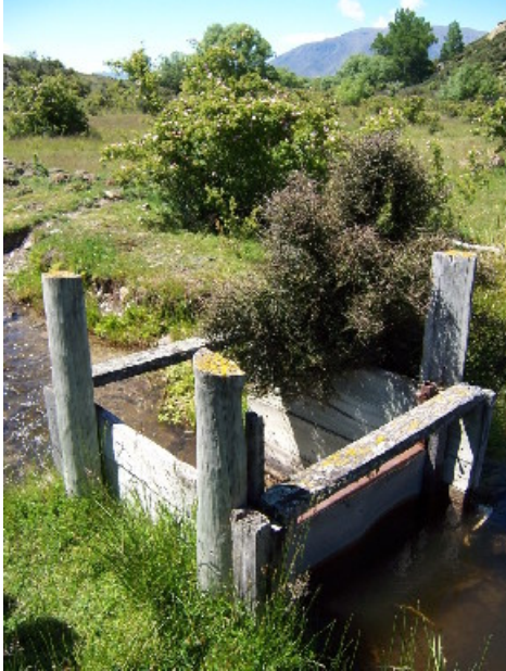
Intake control gates – to be upgraded to meet fish screen requirements
