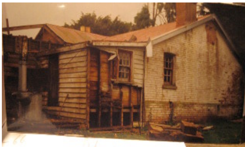
“The Shack” in a derelict state.
