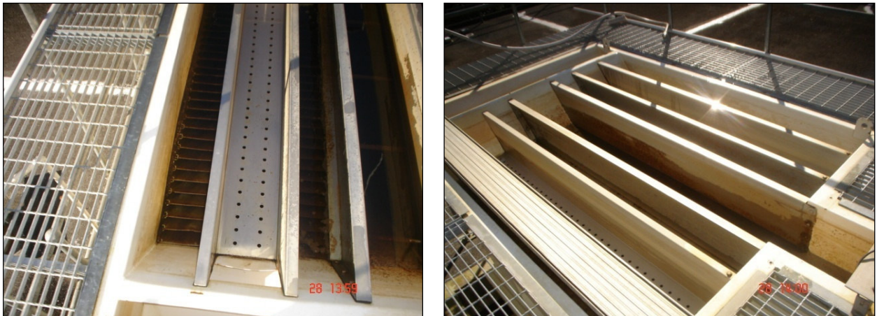
Figure 4-4: View into top of Lamella Clarifier showing inclined plates and overflow channel
