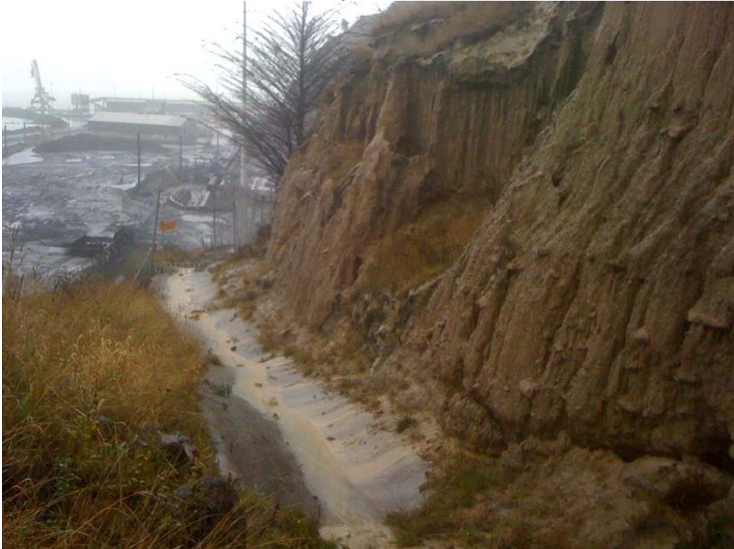
Photo 2: Drain above Coal Yard adjacent to Rill Erosion Loess Area
