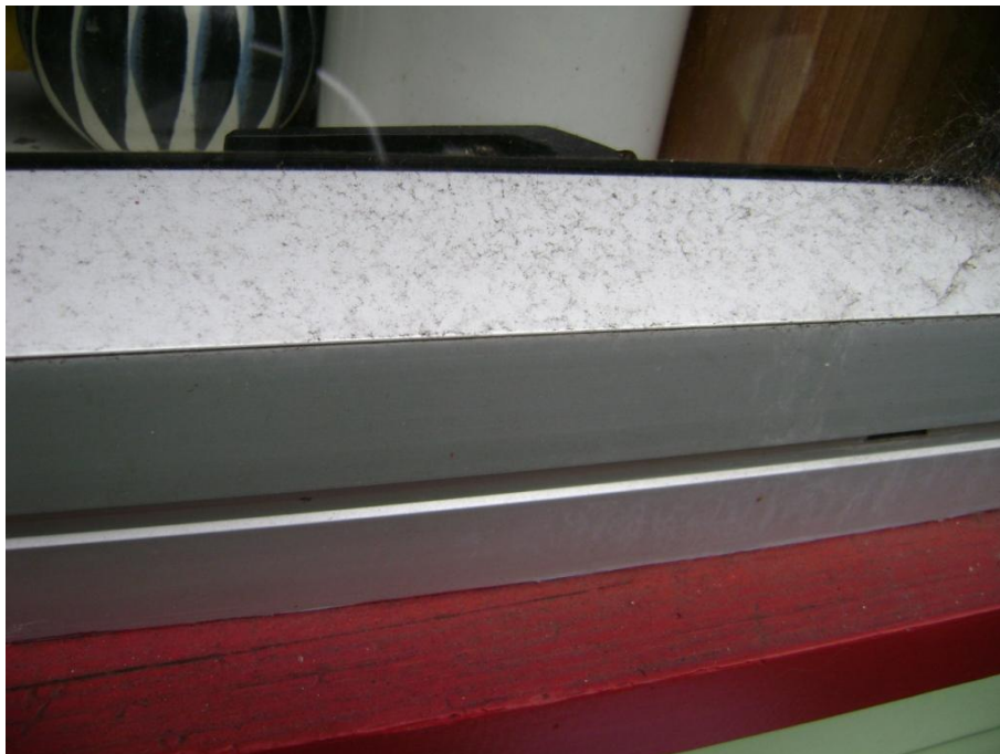
Figure 3: Example of dust accumulation at 4 Randolph Terrace.
