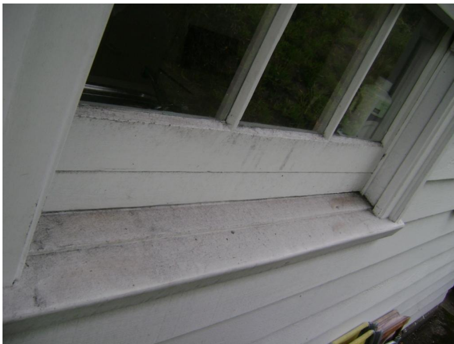
Figure 4: Example of dust accumulation at 2 Gilmour Terrace.
