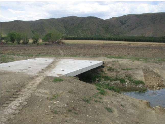
Photo B: Vehicle/Stock Bridge where the pivot crosses Wairepo/Spring Creek. Once finished the bridge will have a gate installed and a fence either side.
