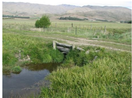
Culvert over stream but the stream is not fenced so stock have access, not a lot of erosion evident though
