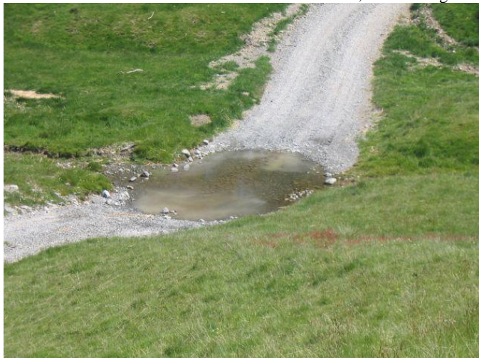
Photo B: Wool wash Creek where the track crosses, additional gravel and planting on the south side is to be completed
