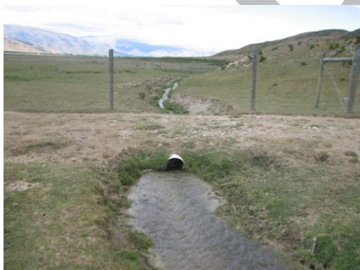
Part of stream within the deer block that needs to be fenced off, note the culvert and also the evident erosion
