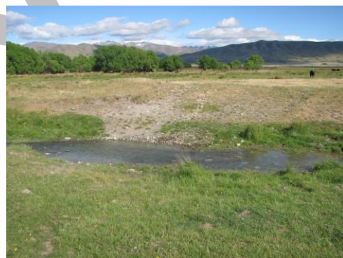
Evidence of erosion, this area should be fenced and culverted to restrict stock access as much as possible
