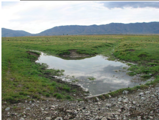
Evidence of a culvert through a stream but notice stock induced erosion
