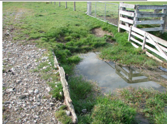
Another culvert where stock have access to water and have caused some erosion
