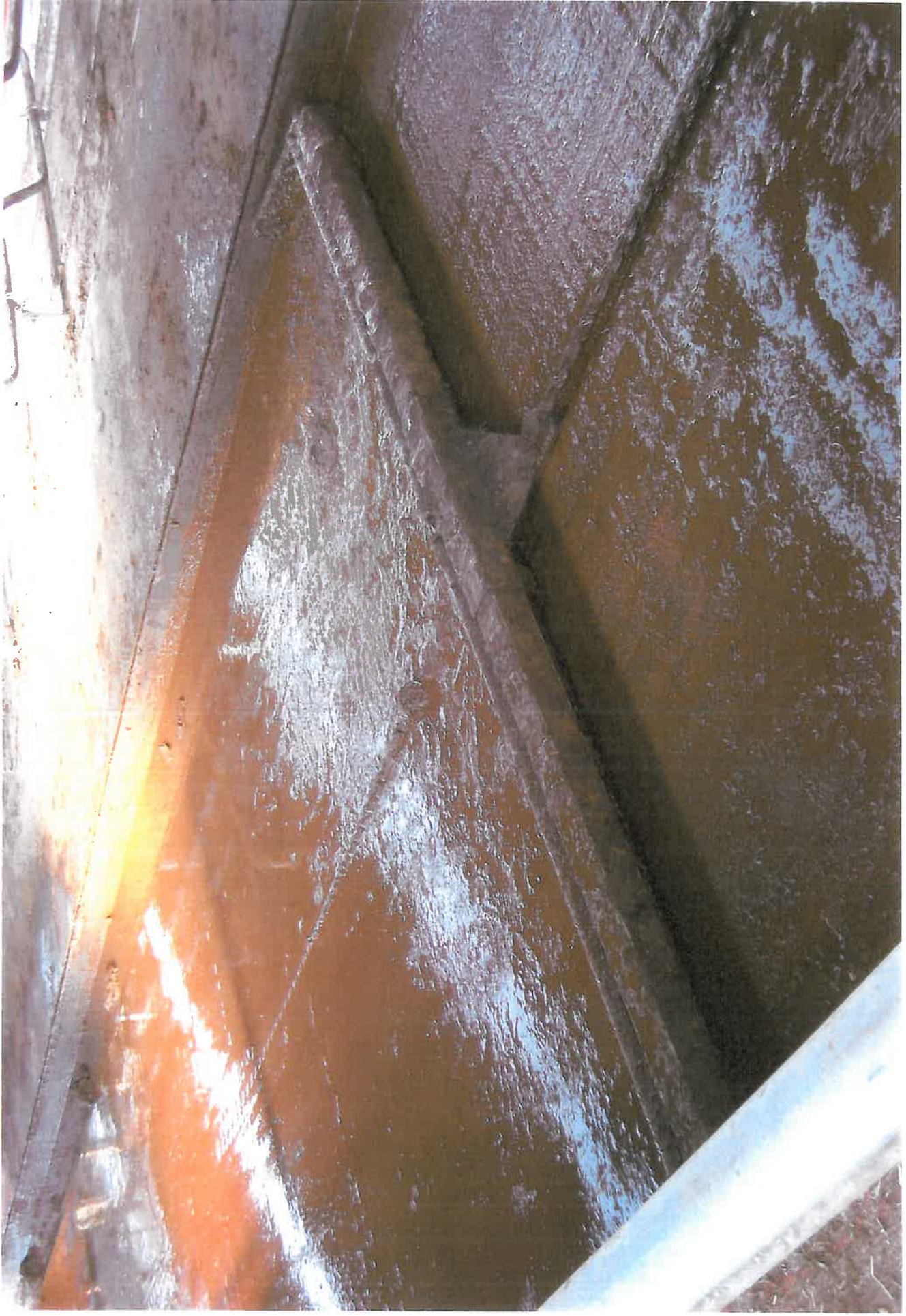
Photo 6: View of an effluent scraper working
