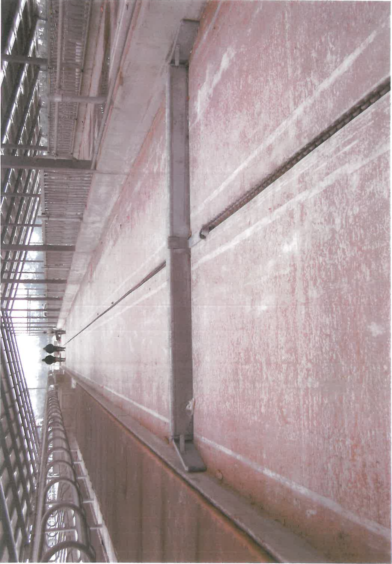
Photo 5: Effluent scraper set in the concrete effluent collection channel AQUALINC
