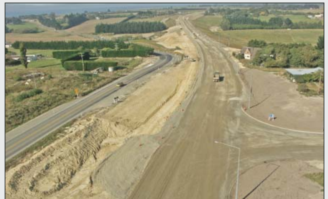
The new 2.6km of state highway just south of Timaru (shown here under construction) is now a significantly safer and more efficient section of road due to an improved alignment, increased lighting and double passing lanes at the south end to improve passing opportunities. The $6 million project opened in May 2005 and finished five months ahead of schedule.
