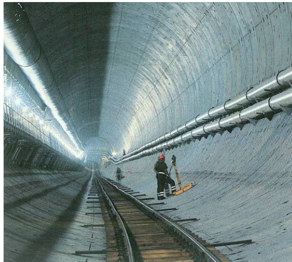
Figure 2-3 Example of precast concrete tunnel lining, which could be used in the alluvial section of the tunnel
