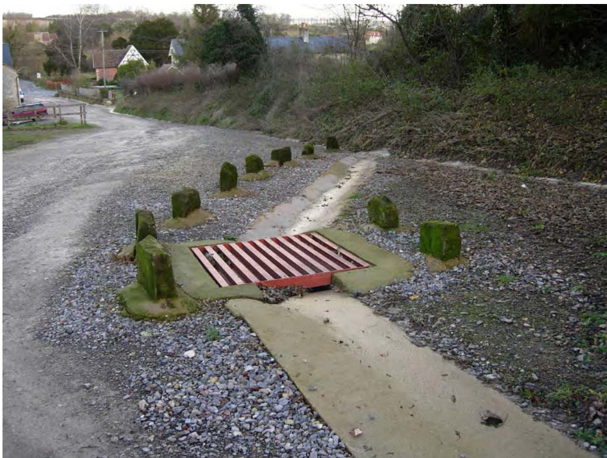
Figure 11 Concrete sediment trap designed to be easily dug out with bucket digger for track runoff
