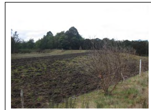
Grazing damage to stop bank
