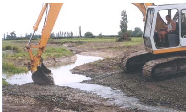
Putting in riffles improves habitat values, and in this case will also act as a weir to raise the water level.
